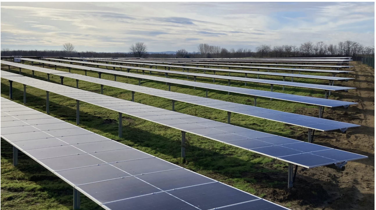
Solar power plant
