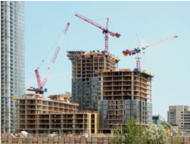
Resident heating and commercial building
