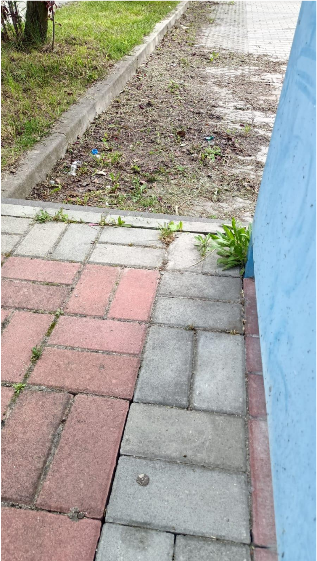
Waste at a corner of a building
