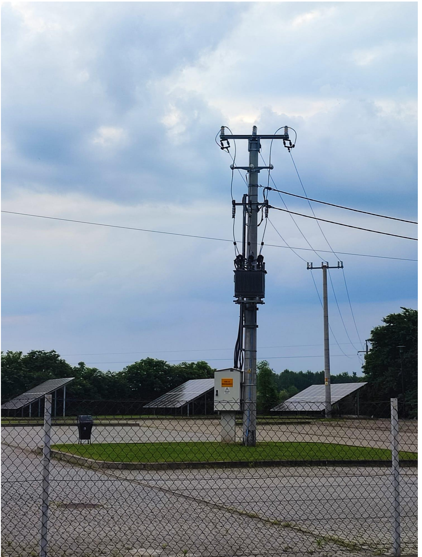
Solar panels near an electrical post – free energy
