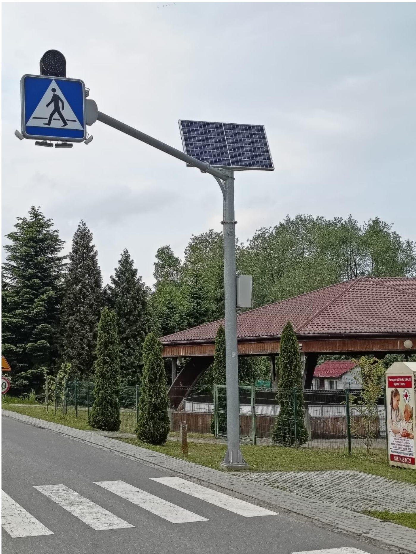
Solar panel on a pedestrian crossing – free light during the night
