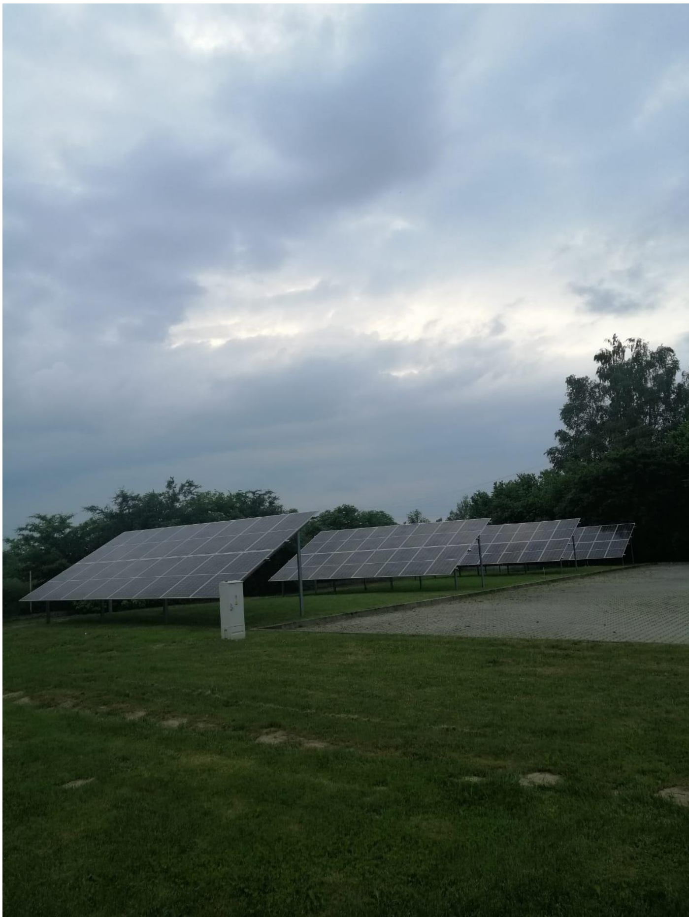
Solar panels – zero emission source of Energy
