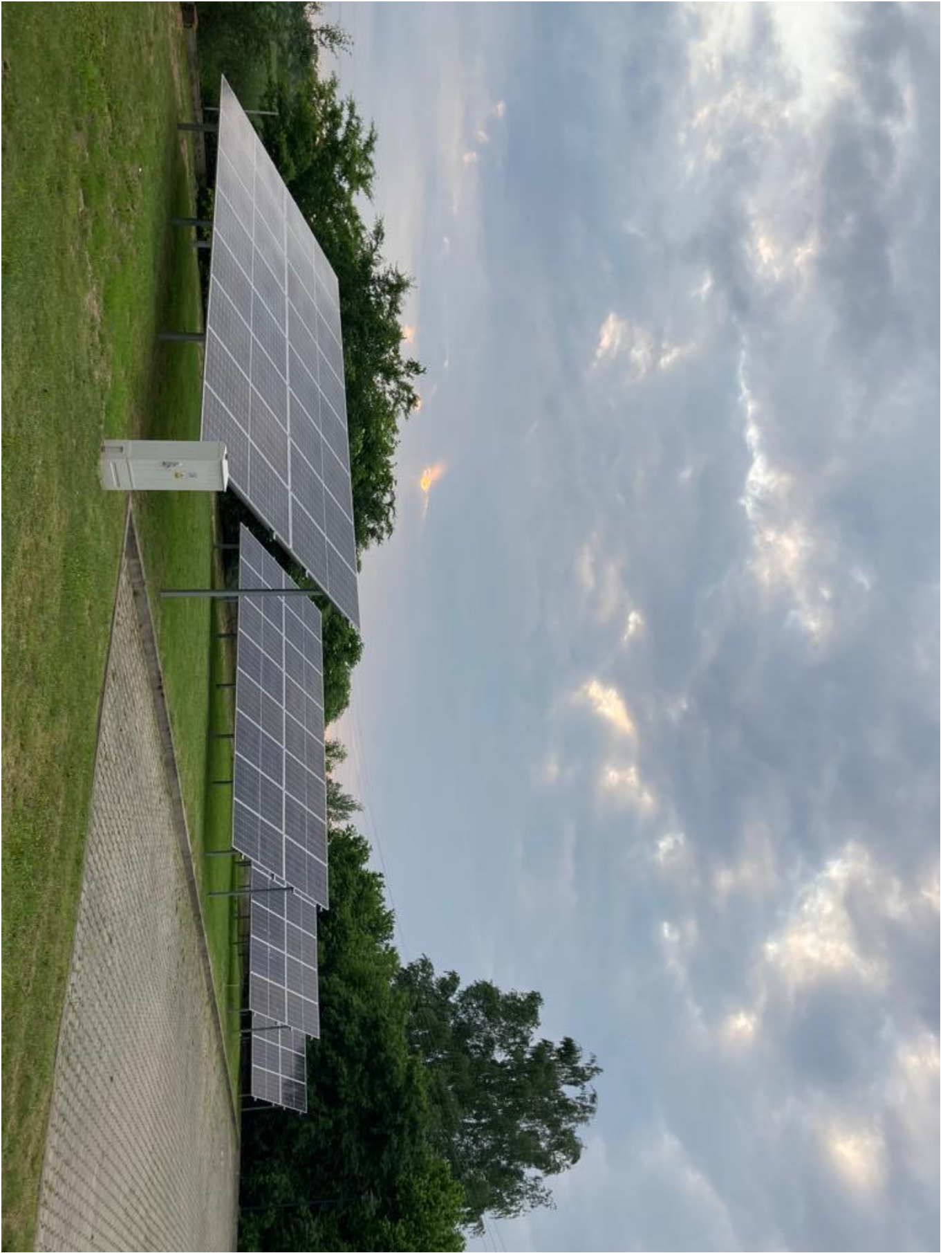
Solar panels – reduce amount of CO 2 in the atmosphere
